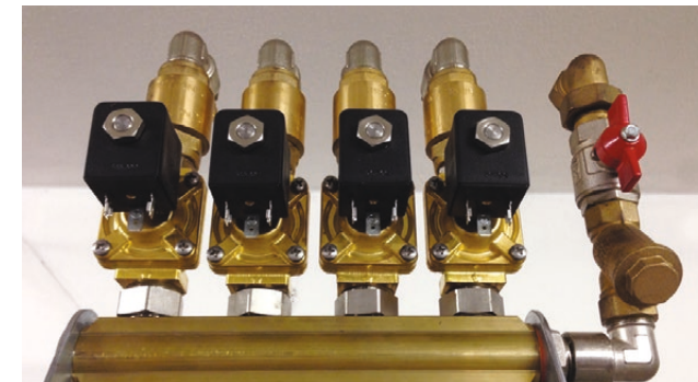
Manual bypass for steam supply in case of black out.
